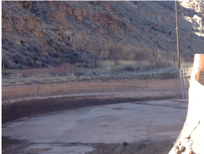
Figure 17. Canal transition zone walls with observed spalling near the top of the wall and near the winter water surface elevations.
