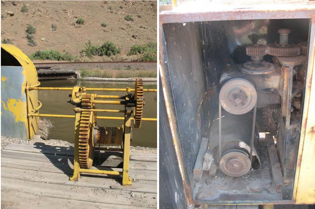
Figure 21. Looking at the manual gate operator (left) and the automated gate operator (right); Grand Valley Project RO&M Exam; July 9, 2008.
