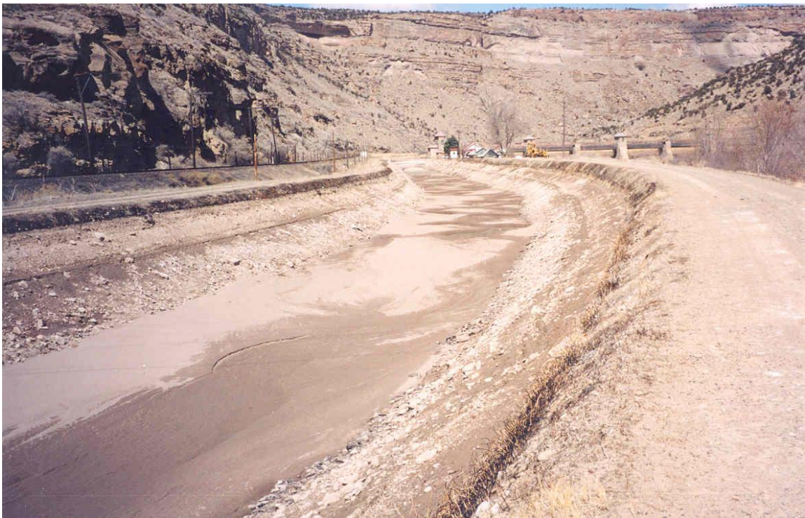
Figure 22. Looking up the canal towards the dam tenders residence at the Roller Dam. Sediment seen in the bottom of the canal is typically sluiced through the Station 22 spillway before and after increased irrigation season flows. Grand Valley Project RO&M Exam; March 18, 2002.
