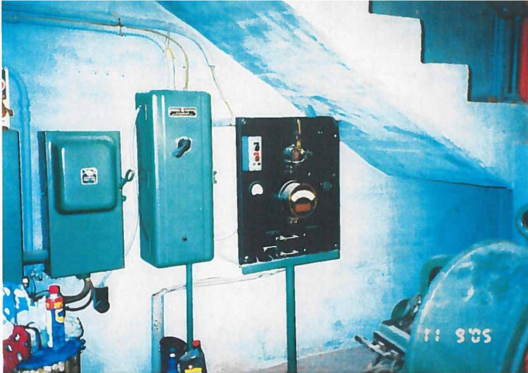
Figure 6. Switch and breaker panels and on/off push button switch (on black panel) for DC power to Grand Valley Diversion Dam, located in power house on the right abutment. Grand Valley Diversion Dam RO&M Exam, Grand Valley Project; November 9, 2005.
