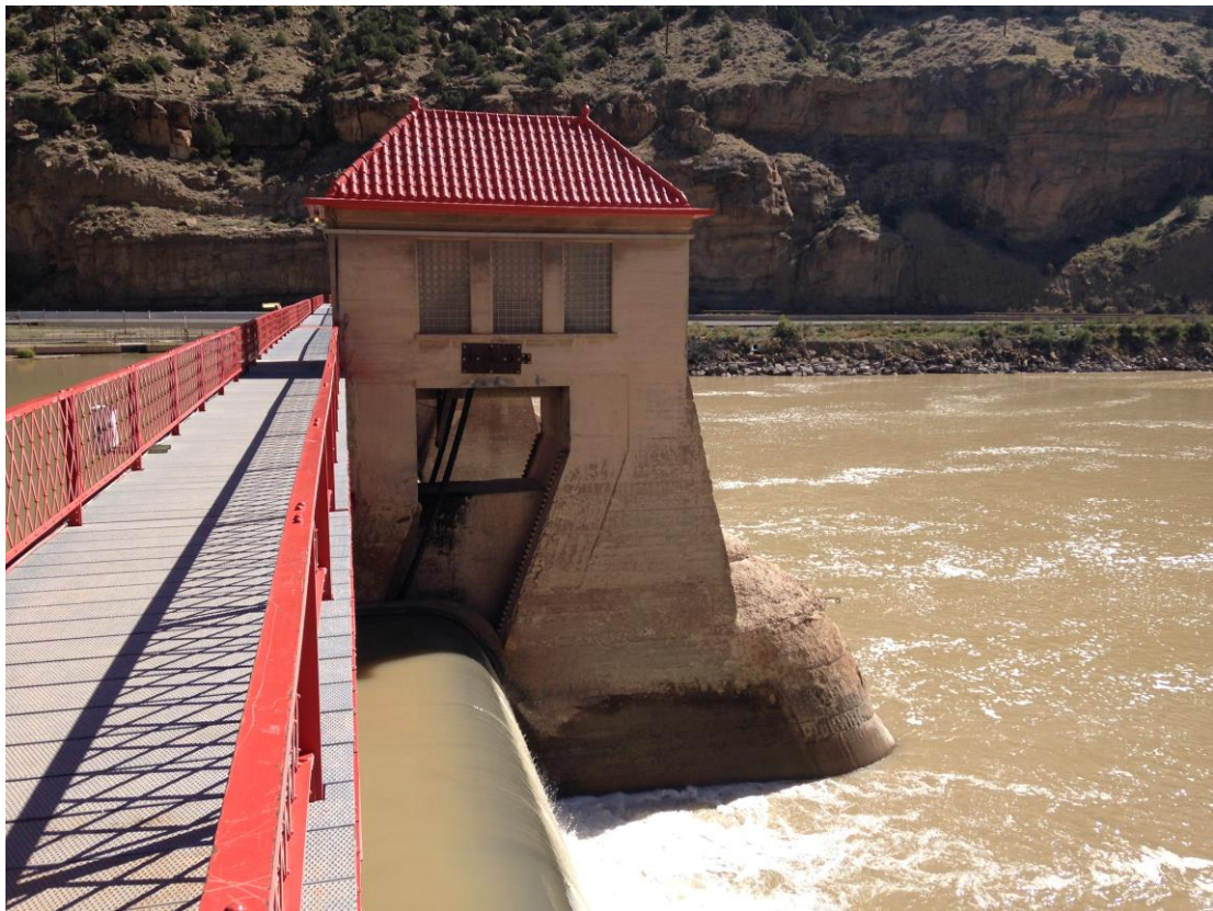
Figure 10. Weathered concrete surface on the downstream side Roller Dam tower.
