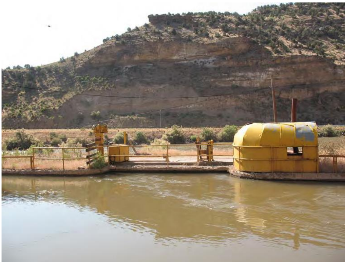
Figure 18. Looking SE across the Canal at the inlet for the Station 22 spillway to the Colorado River, located approximately ½ mile from the Roller Dam. Grand Valley Project RO&M Exam; July 9, 2008.
