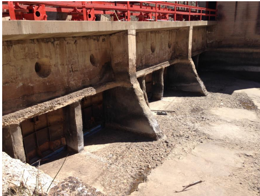
Figure 15. Canal Headgate Structure, downstream side needing concrete repair. Remaining shotcrete from previous rehabilitation efforts can be seen on the support piers.
