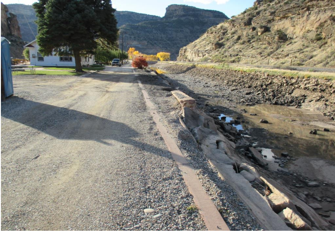
Figure 1. General setting and existing condition of the top 500 feet of the Canyon Canal; looking down canal.
