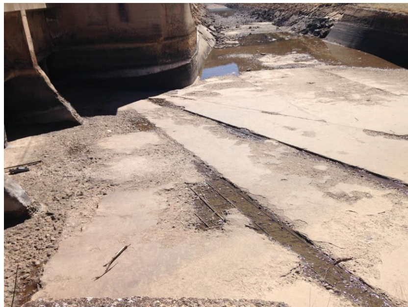
Figure 16. Canal transition zone flooring with observed spalling and exposed rebar.
