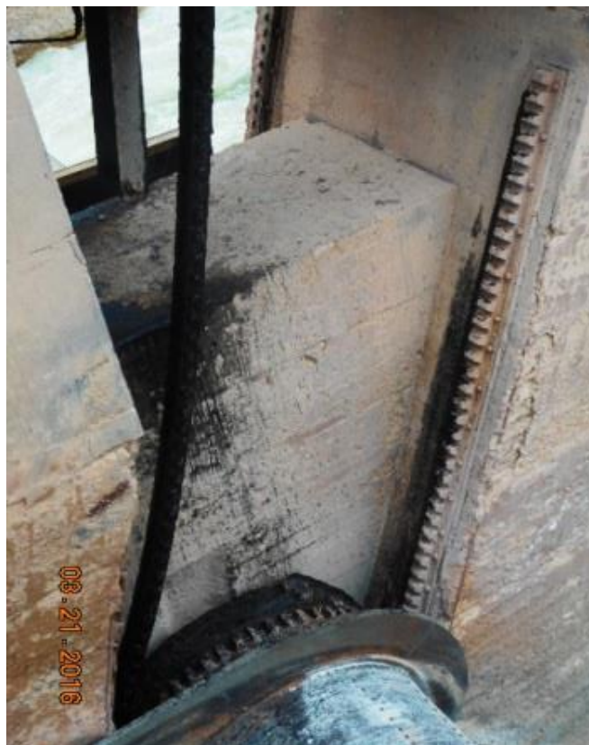
Figure 13. Drive chain (upstream) and track (downstream).
