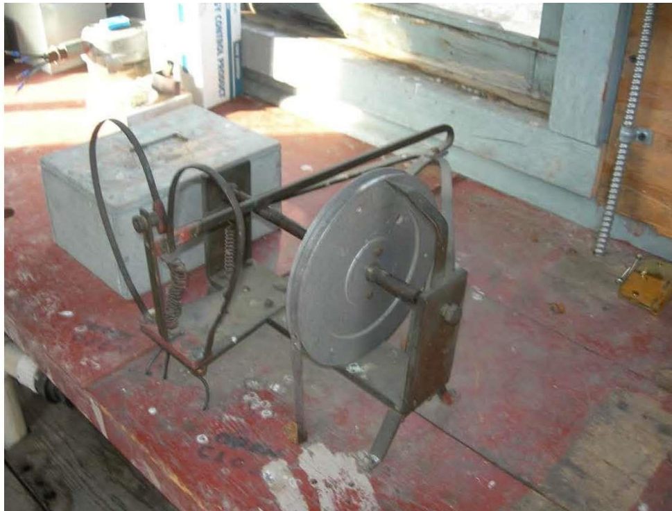
Figure 8. Automation mechanism that regulates flow in canal. Grand Valley Diversion Dam RO&M Exam, Grand Valley Project; November 28, 2011.
