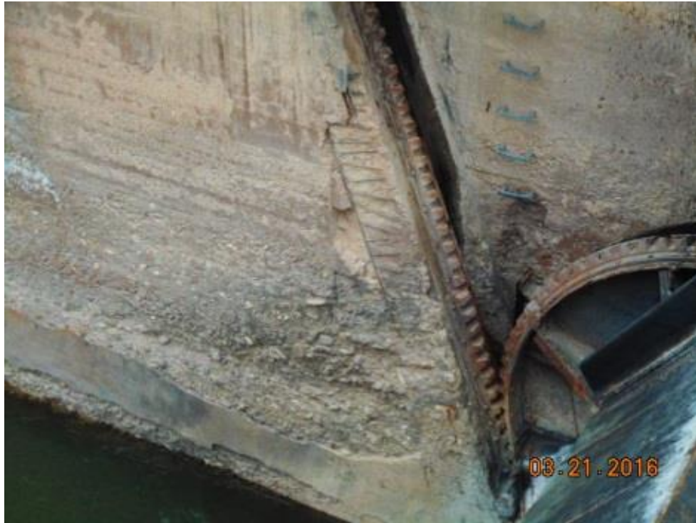
Figure 11. Spalling near the downstream bearing of the roller track (typical).
