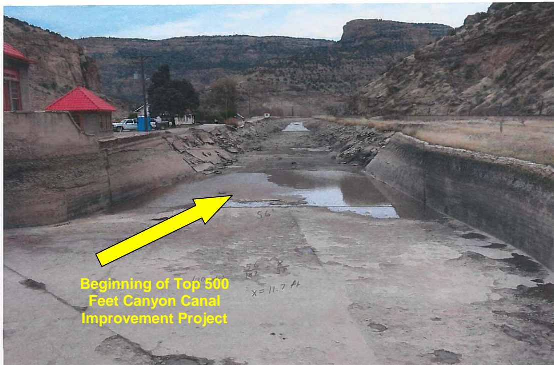
Figure 2. General setting and existing condition of the top 500 feet of the Canyon Canal; looking down canal.
