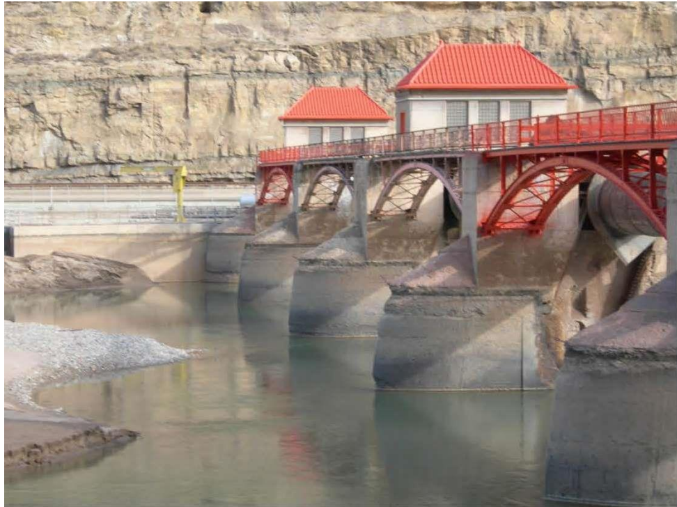
Figure 9. Weathered concrete along upstream footers of Roller Dam. Grand Valley Diversion Dam RO&M Exam, Grand Valley Project; November 28, 2011.
